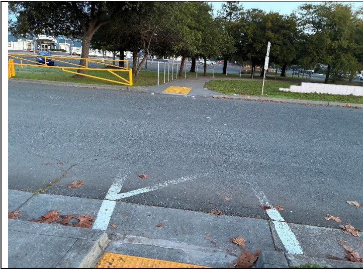
Faded crosswalk across southern entrance to school parking lot
